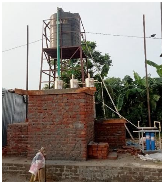
Figure 6.7: Submersible pump near the labor camp
